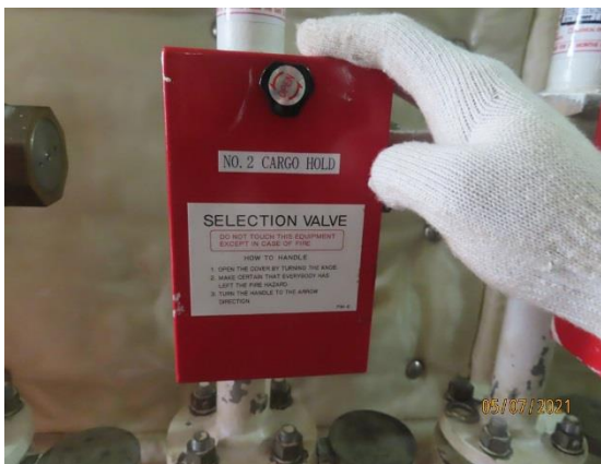
Standby to release Fixed CO2 System in Cargo Hold (Imminent condition)
