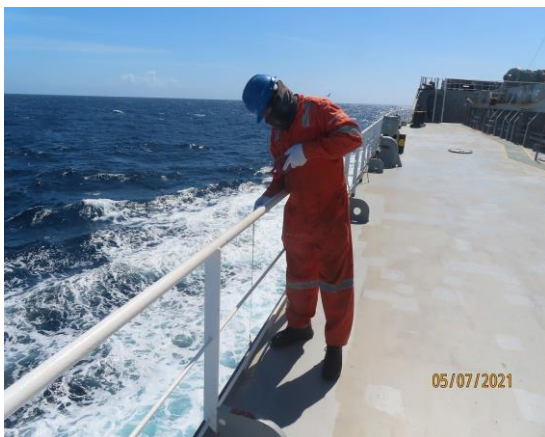
Hull Damage Assessment in way of Frame 160, CHold No. 2 – Port Side
